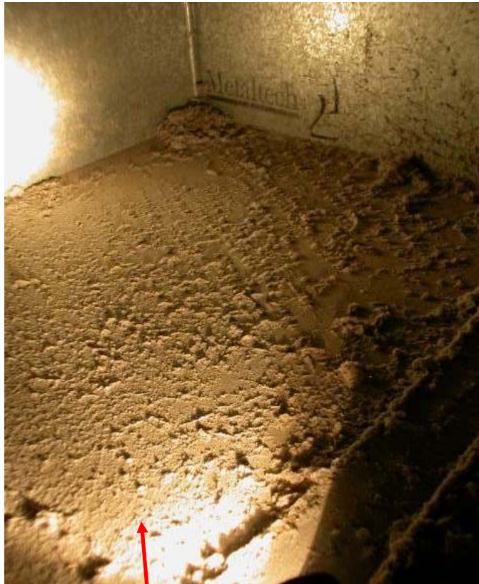
This is a dirty duct
